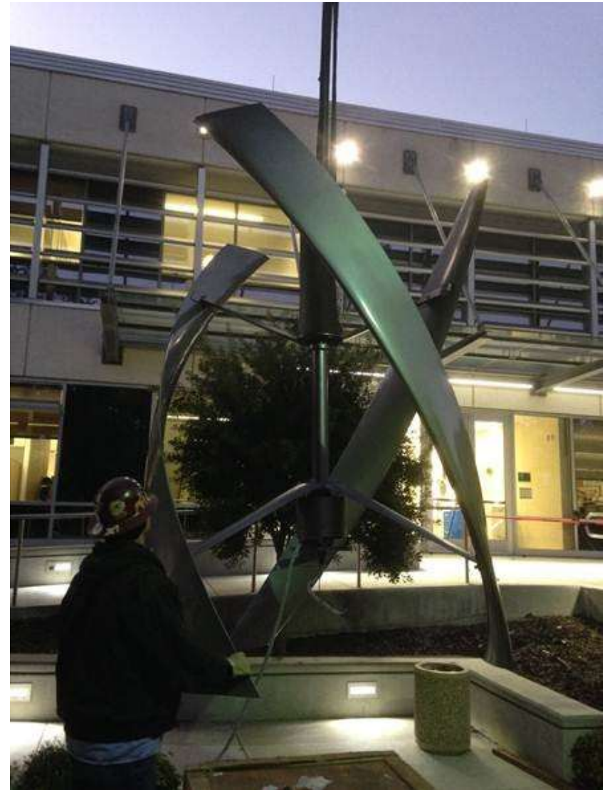
NASA Building 12 turbine installation. Photo from Dave Jager, National Renewable Energy Laboratory
