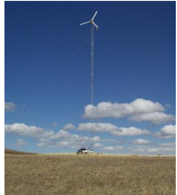
Bergey Excel 10, 10-kW turbine, Klickitat County, Washington Photo by Gwen Bassetti, NREL 26429
