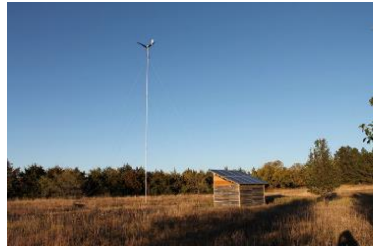
Pika T701 turbine in Gorman, Maine Photo from Pika Energy, NREL 31728
